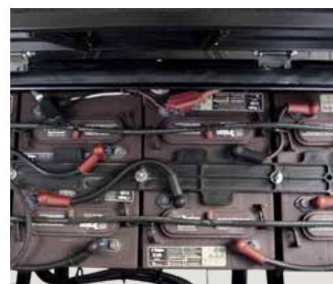
Automatic Battery Watering System
